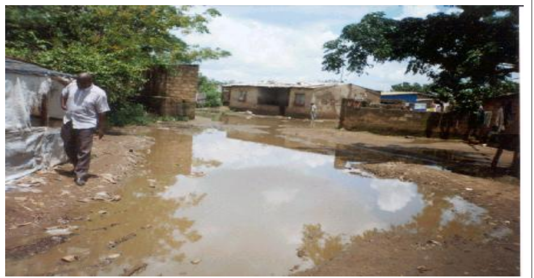
The result of poor or no drainage— Flooded and Damaged roads in Lusaka's Kanyama Compound
