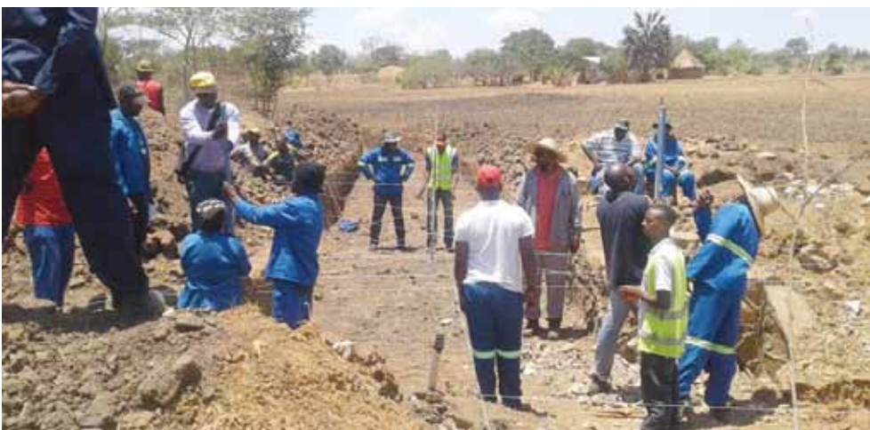
Road Construction and Maintenance Supervision Course students on site installing a double barrel 900mm culvert in Kanakantapa.
