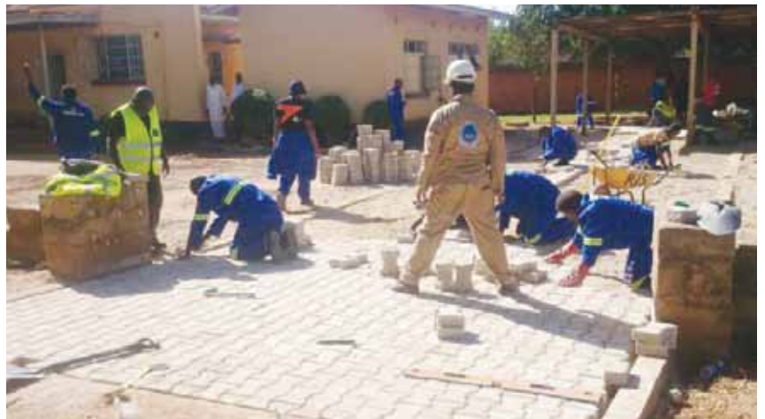
The Brick Paving Technology Course held in Kabwe and conducted with 26 Contractors paved part of the Kabwe Railway Clinic as part of their training.
